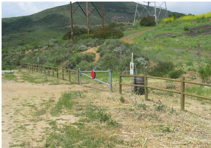
The new peeler pole fencing installed at Black Mountain Open Space Park.
