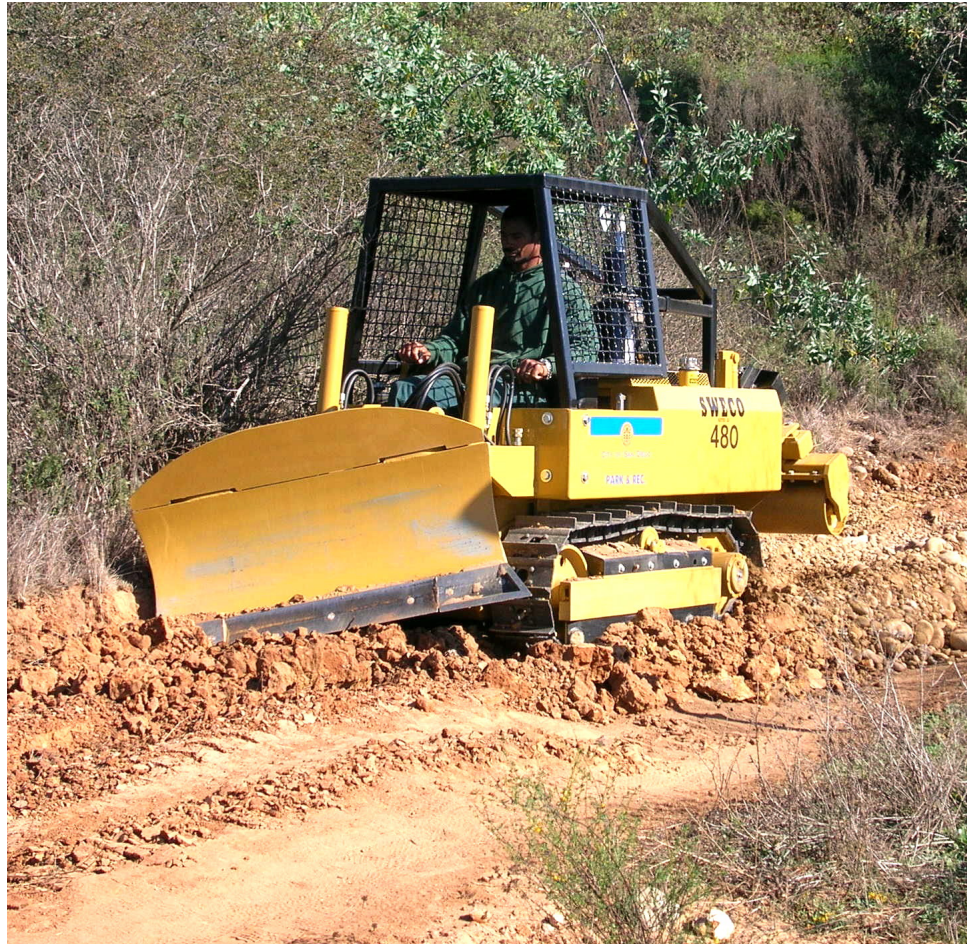
City Ranger John Garwood working the new Sweco trail building tractor on the "Upper Cobbles" trail north of the waterfall in Peñasquitos Canyon Preserve.
