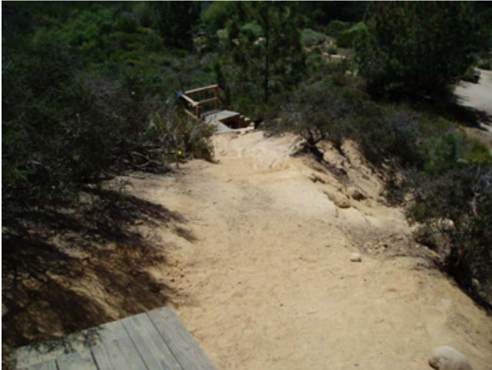
Now, if we only had a middle! Stairs under construction in Crest Canyon. Black Mountain Open Space Park Senior Ranger Ed Christenson also manages the Crest Canyon Preserve, on the south side of the San Dieguito River Valley, west of I-5. See inside for completion photo.
